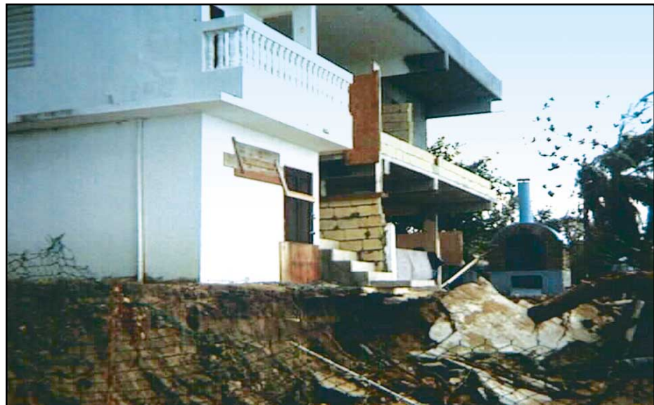
Figure 2-17 Hurricane Georges (1998). Coastal building in Puerto Rico damaged by storm surge and waves.
