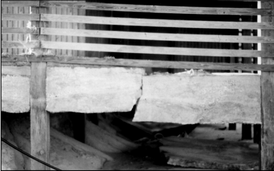
Figure 2-7 March 1989 northeaster. This plain concrete perimeter grade beam cracked in several places.
