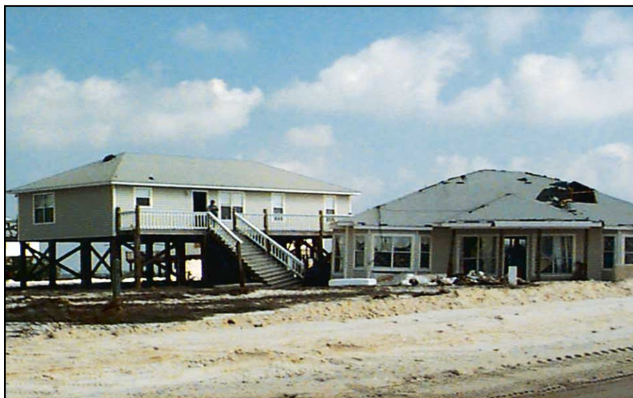
Figure 2-21 Hurricane Georges (1998), Dauphin Island, Alabama. As a result of erosion, scour, and inadequate pile embedment, the house on the right was washed off its foundation and into the house on the left.
