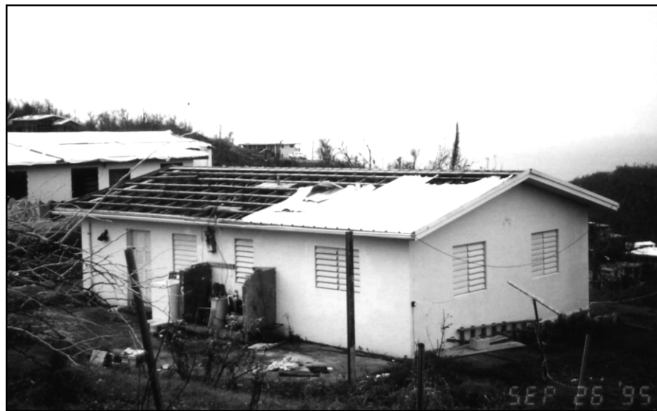
Figure 2-14 Hurricane Marilyn (1995). This house lost most of the metal roof covering. Neighbors stated that the house also lost its roof covering during Hurricane Hugo, in 1989.
