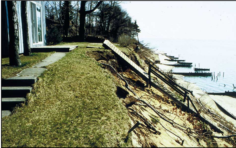
Figure 2-28 August 1988. Erosion along the Lake Michigan shoreline at Holland, Michigan, resulting from high lake levels and storm activity (photo courtesy of Mark Crowell).
