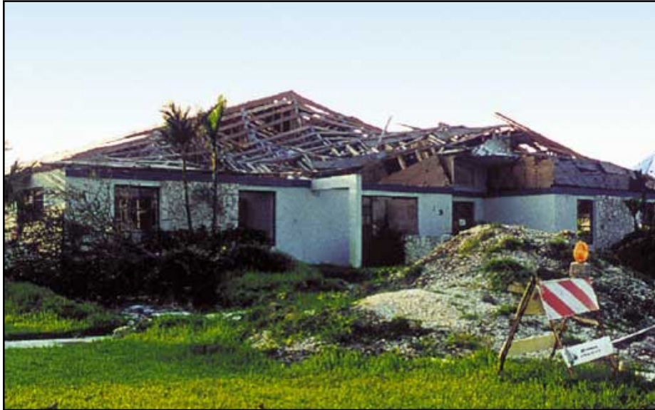
Figure 2-13 Hurricane Andrew (1992). Roof structure failure due to inadequate bracing.
