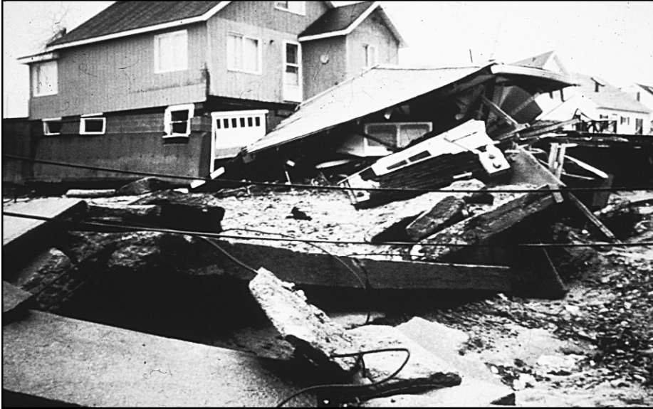
Figure 2-4 October 1991 northeaster damage to homes at Scituate, Massachusetts. Photograph by Jim O'Connell.
