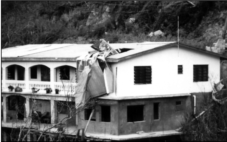
Figure 2-15 Hurricane Marilyn (1995). The roof of this house was penetrated by a large wind- driven missile (metal roof covering).
