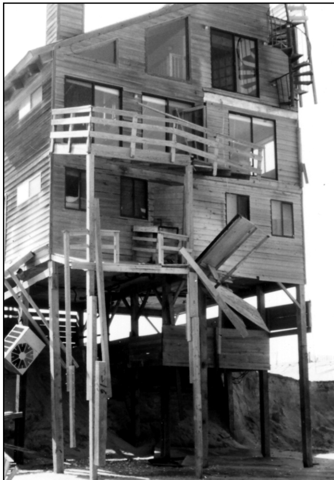
Figure 2-8 March 1989 northeaster. Although this house seems to have lost only several decks and a porch, the loss of supporting soil leaves its structural integrity in question.
