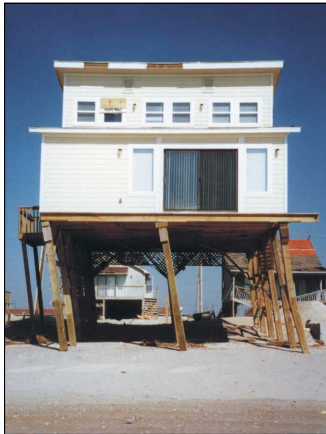
Figure 2-16 Hurricane Fran (1996). Many oceanfront houses built before the enactment of the 1986 North Carolina State Code were found to be leaning or destroyed.
