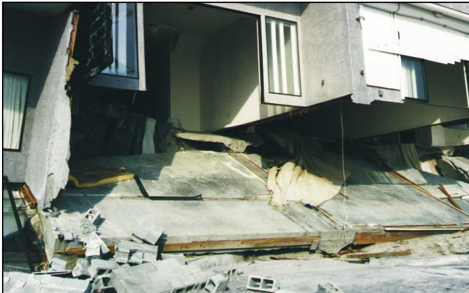
Figure 2-20 Hurricane Opal (1995), Bay County, Florida. Building damage from erosion and undermining.
