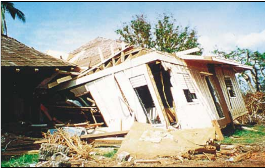
Figure 2-24 Hurricane Iniki (1992). Non-elevated house at Poipu Beach that floated off its foundation and was pinned against another house and destroyed by waves.
