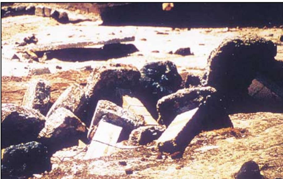
Figure 2-25 Hurricane Iniki (1992). Undermining of shallow footings supporting columns at Poipu Beach due to lack of sufficient embedment below erosion level.
