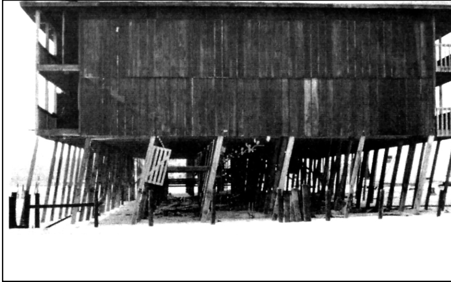
Figure 2-19 Hurricane Frederic (1979). Effects of wind and water forces on unbraced pile foundation.
